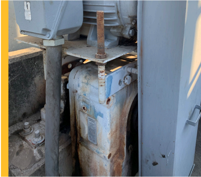
The existing belt-driven system with an obsolete gear reducer was inefficient and laborious to maintain, requiring frequent inspections by two technicians.
